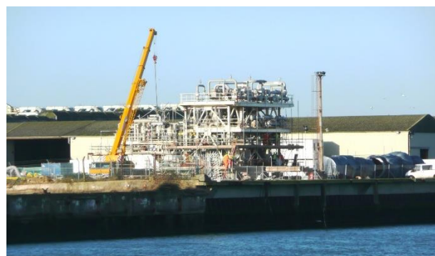
Figure 6: View of Jeld-Wen quay being used in 2014 for offshore assembly and load-out using mobile crane on the quayside
