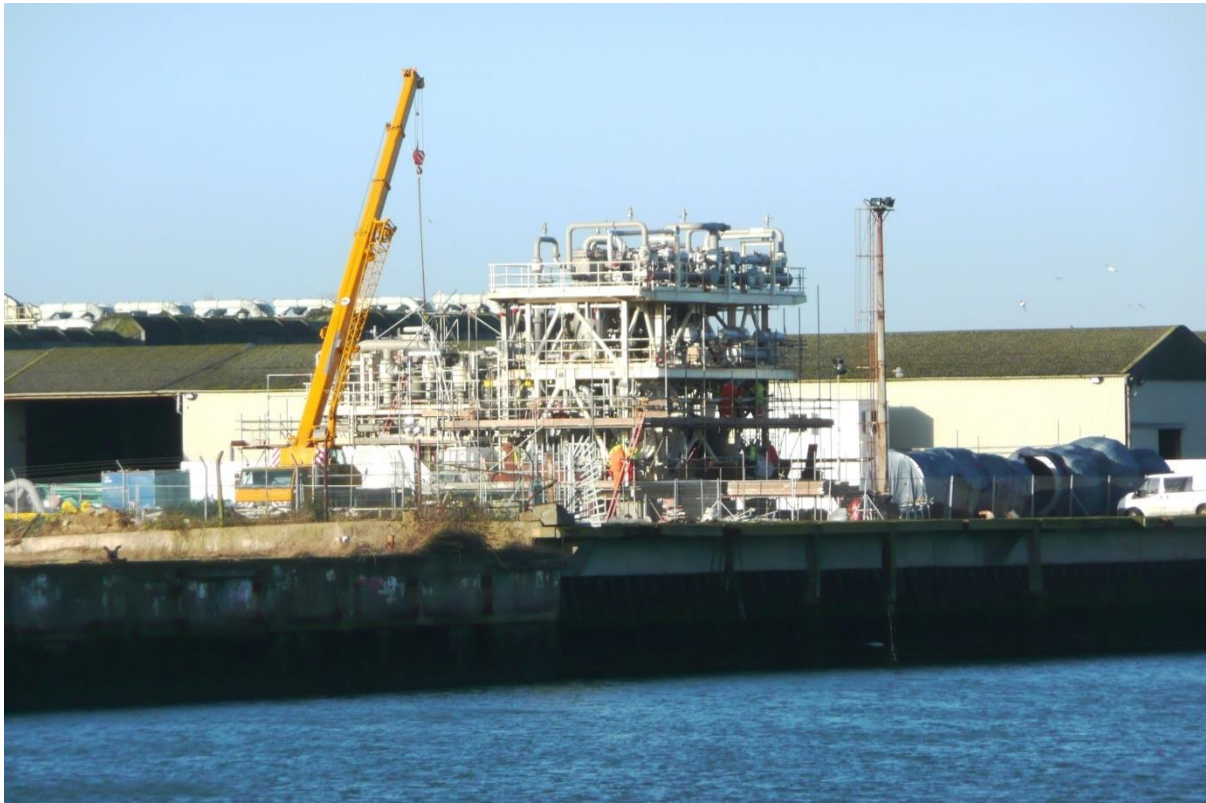
Figure 48: View of Jeld-Wen quay being used in 2014 for offshore skid frame assembly prior to load-out using a 1000Te mobile crane on the quayside [image courtesy of Technicus Consulting]
